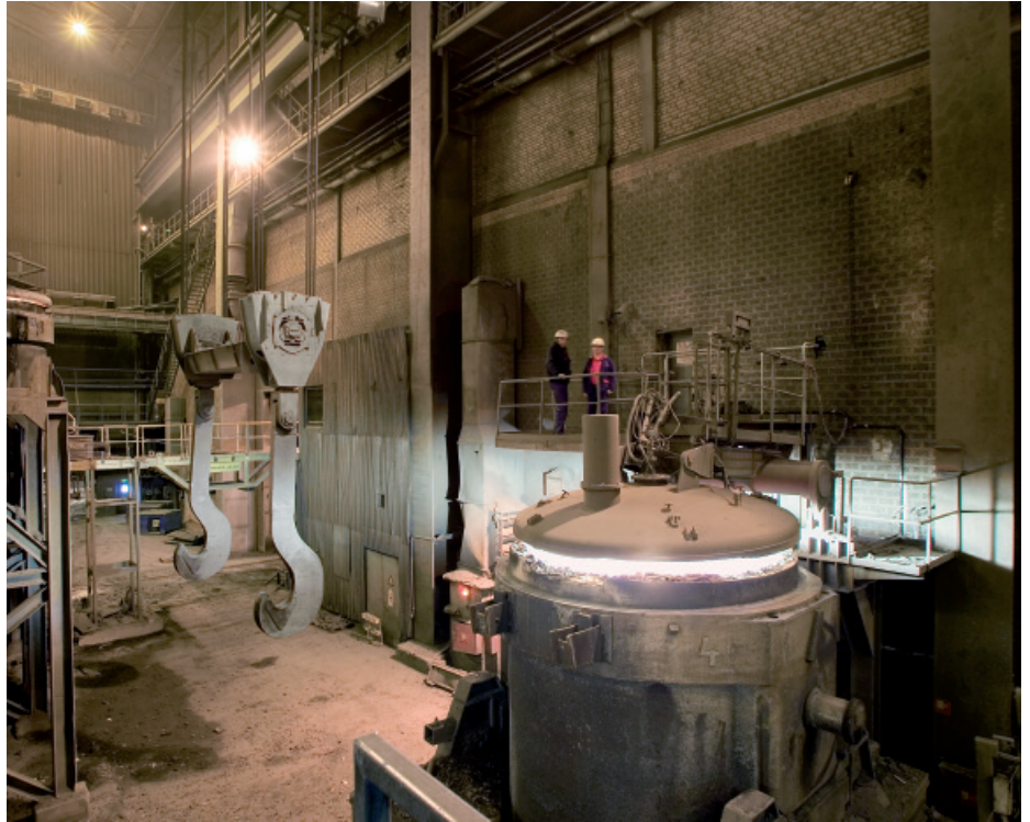
Flameless oxyfuel in vessel preheating allows for shorter tap-to-tap cycles and lowers costs.
